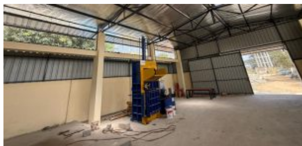
Fig: Heat resilient features inside the DWCC
