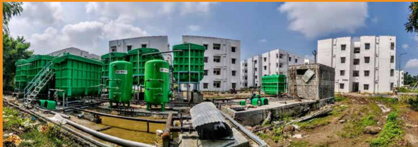
Figure 6: Decentralised wastewater treatment plan in low-income housing facility in Warangal
